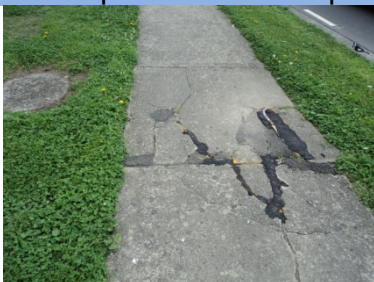
Hazards likely to cause trips and falls
