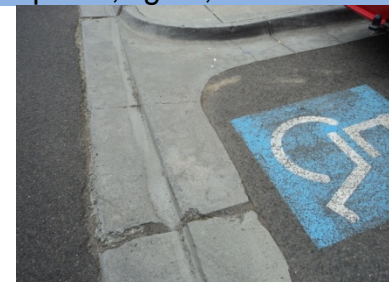
No rollover kerb behind accessible car park
