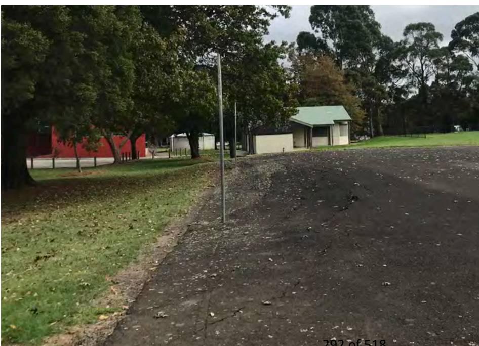
The court surface has deteriorated at the southern end, and is unsuitable for use in its current condition.
