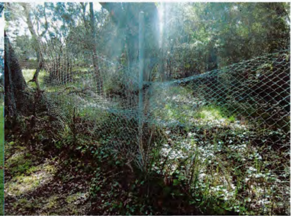
Photograph 4: Fence in disrepair
