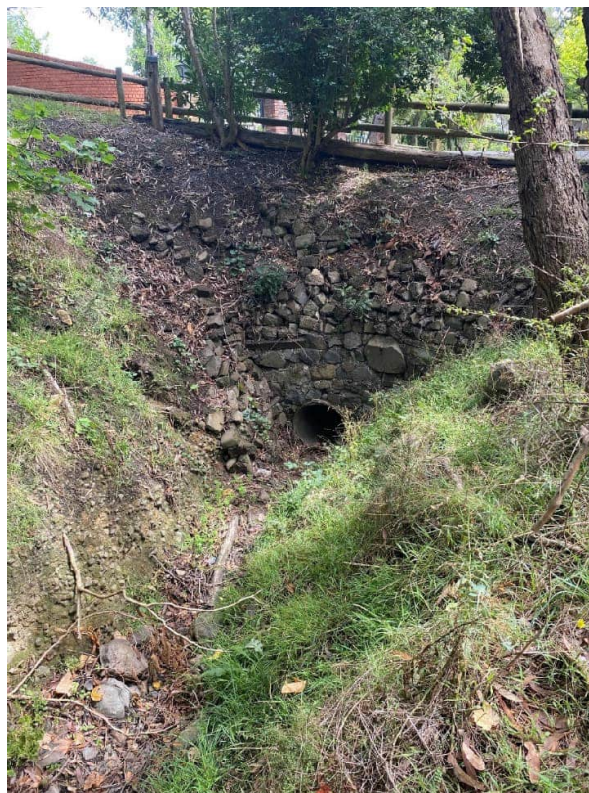
Figure 7.10 Gully blocked by driveway fill, Olivebank Road, Ferntree Gully. Colluvium exposed in side of gully.
