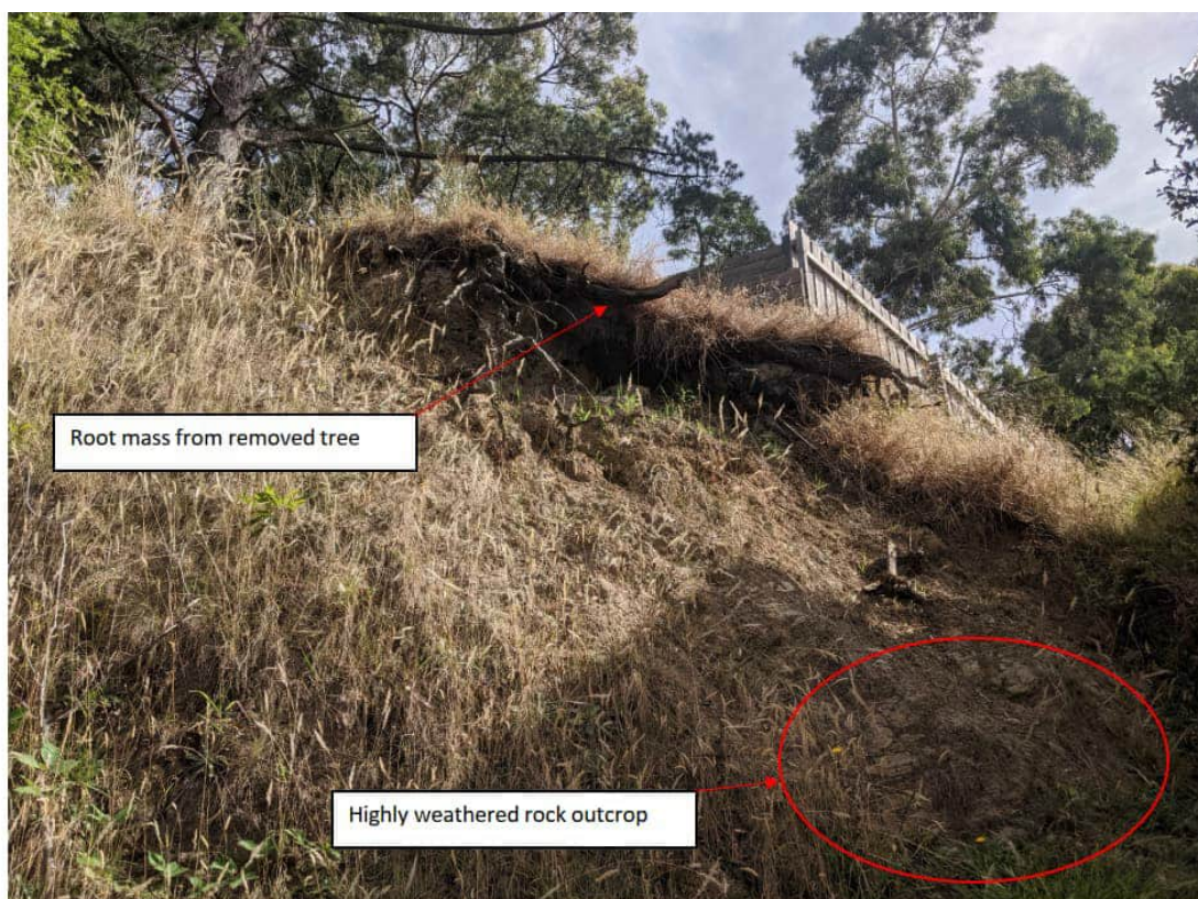
Figure 7.1 Landslide scarp at 1015 Burwood Highway (photograph taken in 2021)
